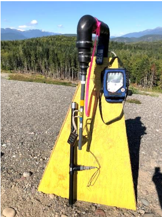
Photo 1 – LFG Monitoring - Vent #3
