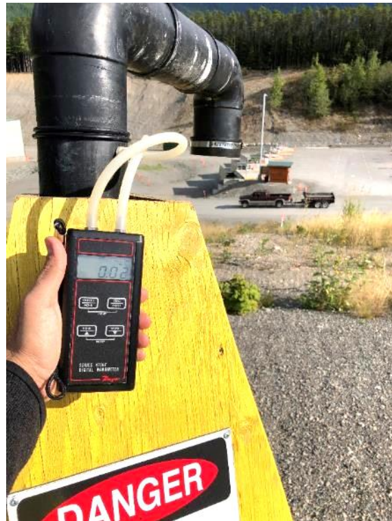
Photo 2 – Capped Vents Gas Pressure monitoring
