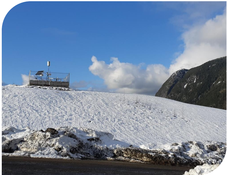
Figure 1 Landfill gas flare at the closed Thornhill Landfill.
