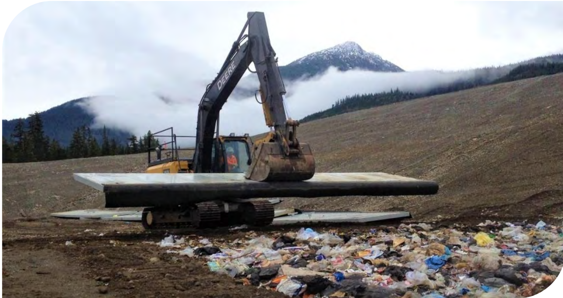
Figure 4 Placement of RIG plates as alternative daily cover at the landfill at Forceman Ridge WMF.
