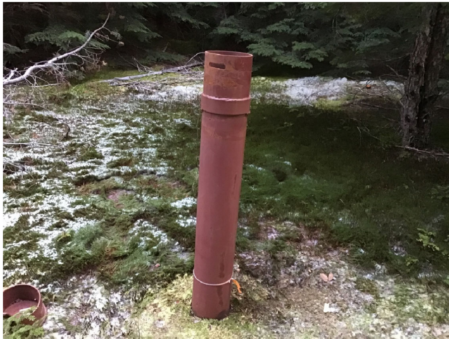
Photo 61: Forceman Ridge Waste Management Facility MW-10, well head, December 1, 2022
