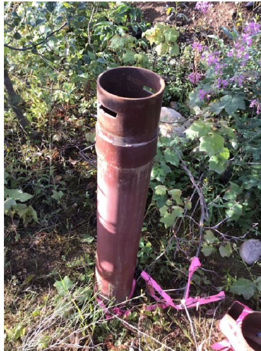
Photo 67: Forceman Ridge Waste Management Facility MW-12, well head, August 31, 2022
