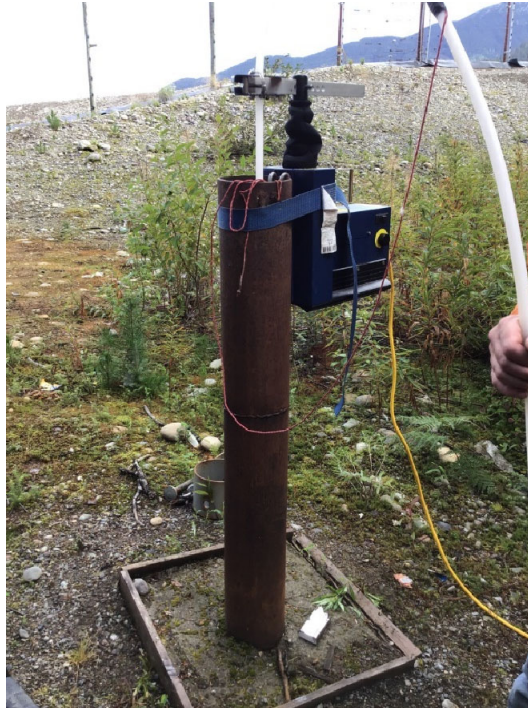
Photo 78: Forceman Ridge Waste Management Facility MW-15, well head, August 31, 2022
