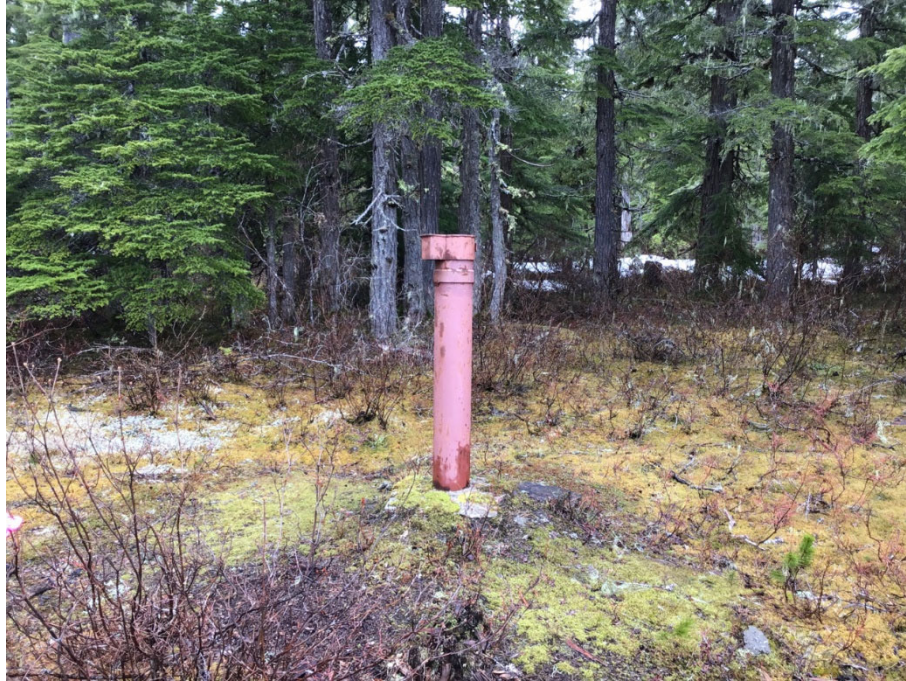
Photo 46: Forceman Ridge Waste Management Facility MW-07, well head, March 25, 2022
