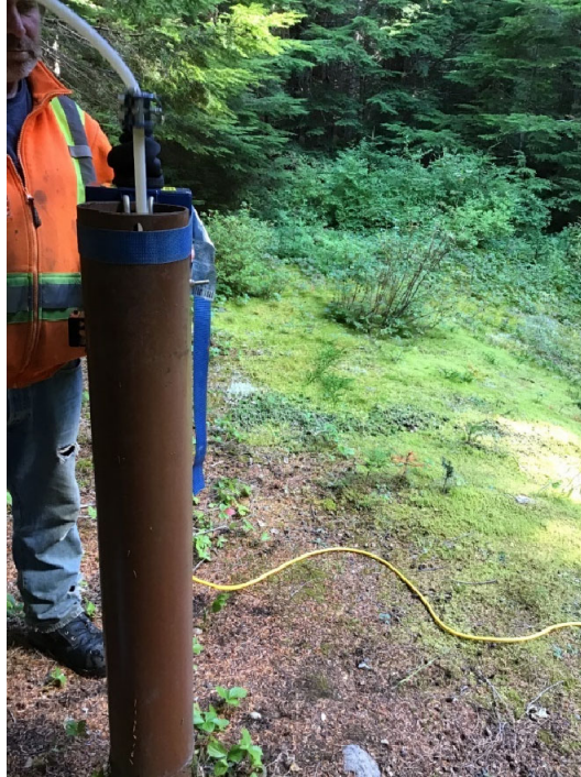
Photo 36: Forceman Ridge Waste Management Facility MW-04, well head, August 31, 2022
