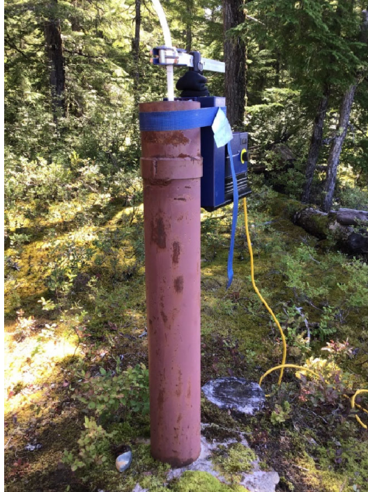
Photo 48: Forceman Ridge Waste Management Facility MW-07, well head, August 31, 2022
