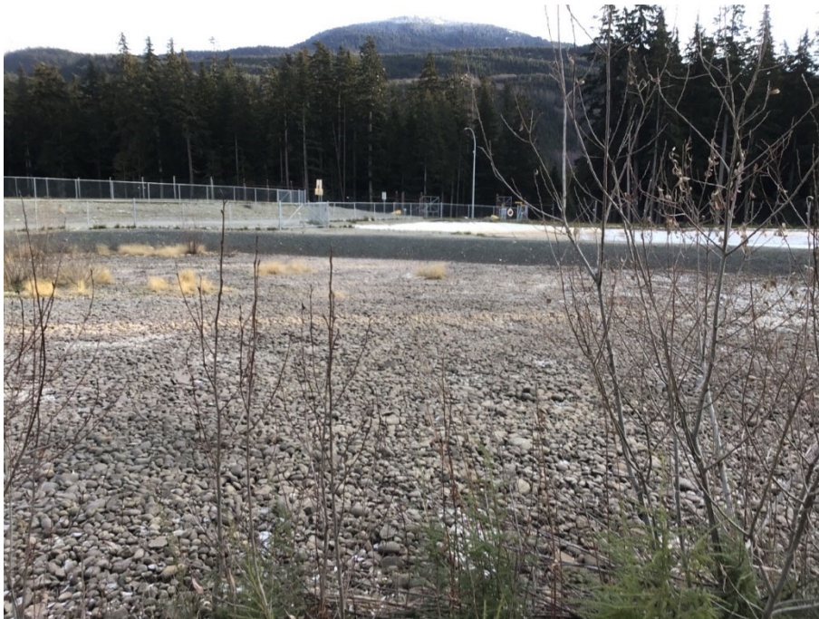
Photo 87: Forceman Ridge Waste Management Facility Sand Filter, surrounding area looking NE, December 1, 2022
