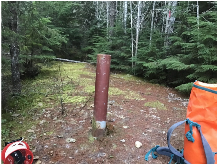
Photo 65: Forceman Ridge Waste Management Facility MW-11, well head, December 1, 2022
