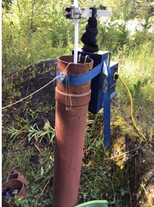
Photo 52: Forceman Ridge Waste Management Facility MW-08, well head, August 31, 2022
